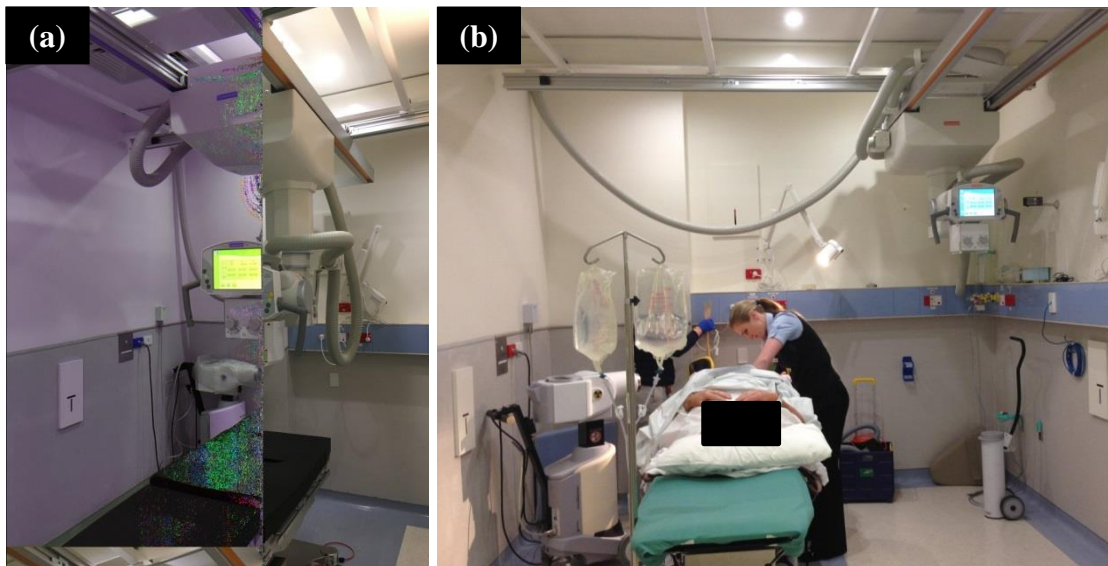
Figure 7.5. (a) The treatment room ceiling suspended x-ray system used for pre-treatment imaging and (b) the system parked out of the way during a clinical case.
