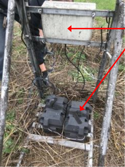
Electronics & batteries behind panel
