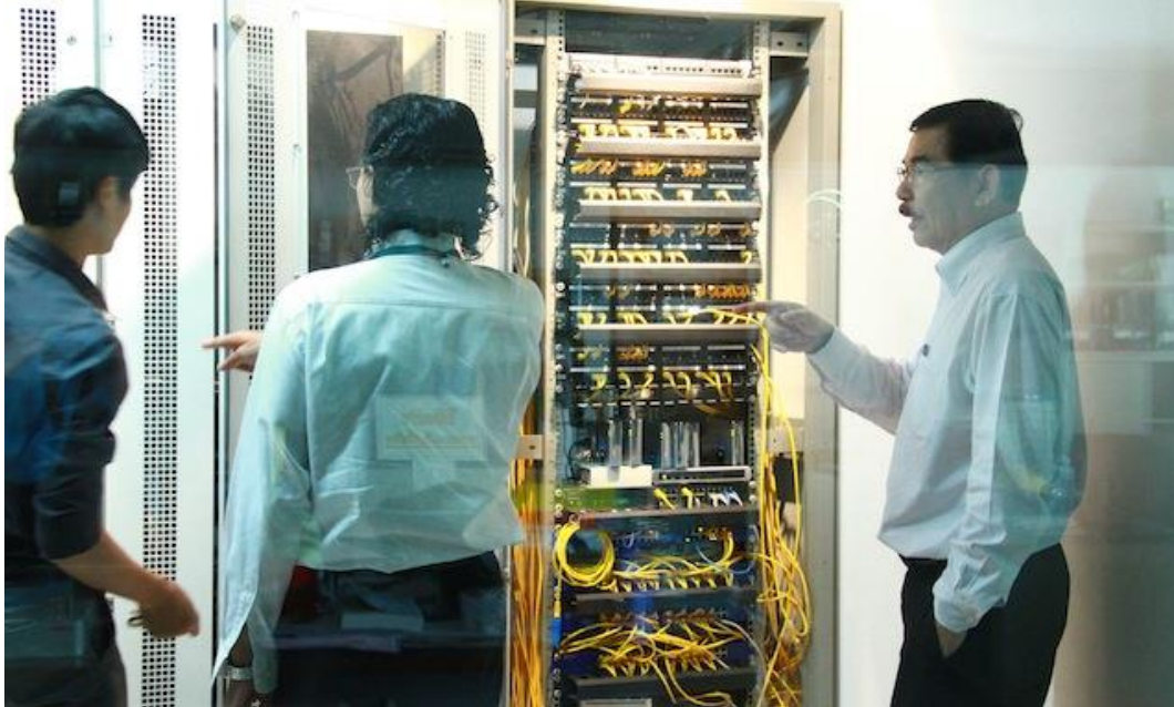
Image 5.1: Testing the Server
