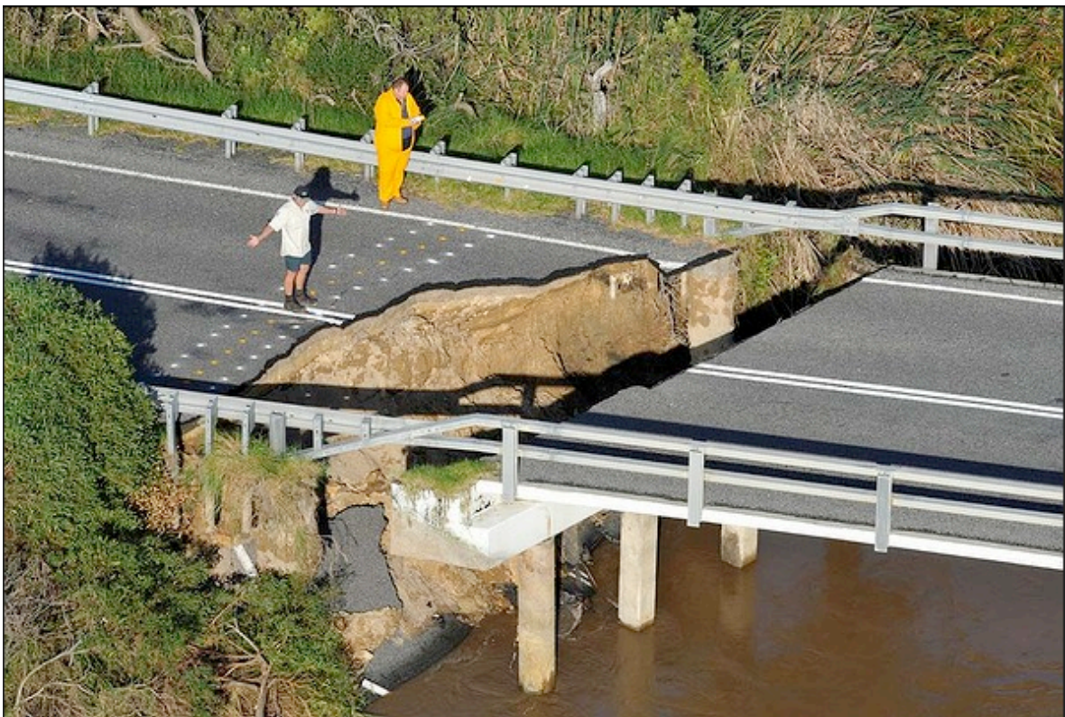
Figure 5.2 – 23 March 2011. The damaged Darby Bridge. Photo: Justin McManus.
