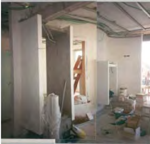
4. Dadush residence, curved wall with holes and cantilevers to become: the toilet room, shelves systems and sofa as a nook looking at the sea, under construction, 1994.
