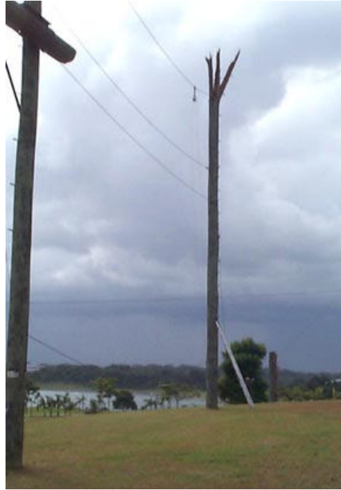
Figure 2.2: Pole destruction by lightning strike [6]
