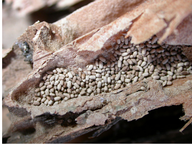
Figure 2.1: Wood deterioration as a result of termite attack [5]
