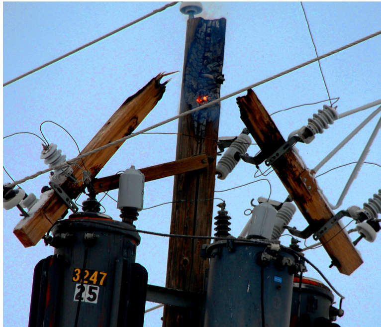
Figure 2.4: Pole-top fire event in Southmoor distribution line [8]
