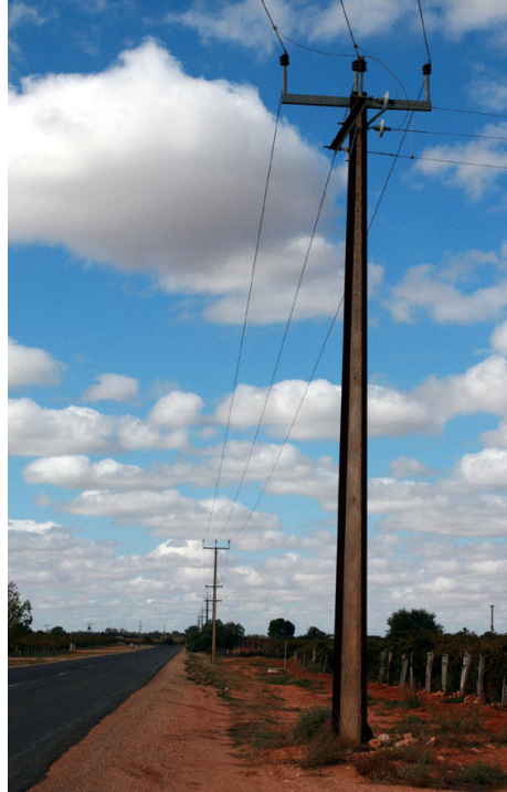
Figure 1.2: Stobie pole in South Australian electrical distribution network [2]
