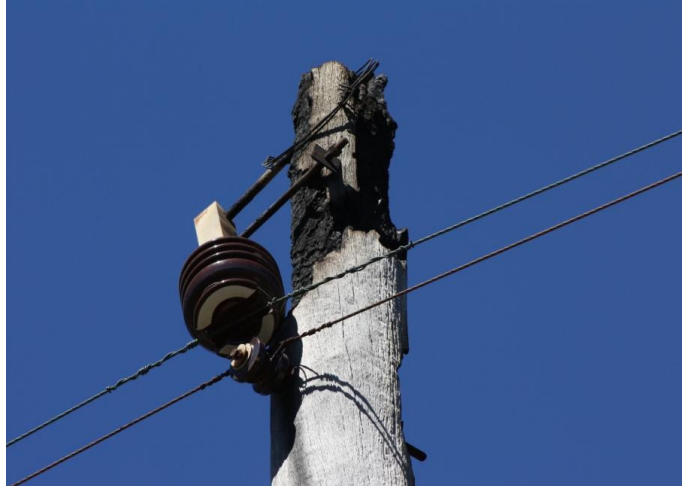
Figure 1.4: Pole-top fire in Dunsborough electrical distribution network [4]
