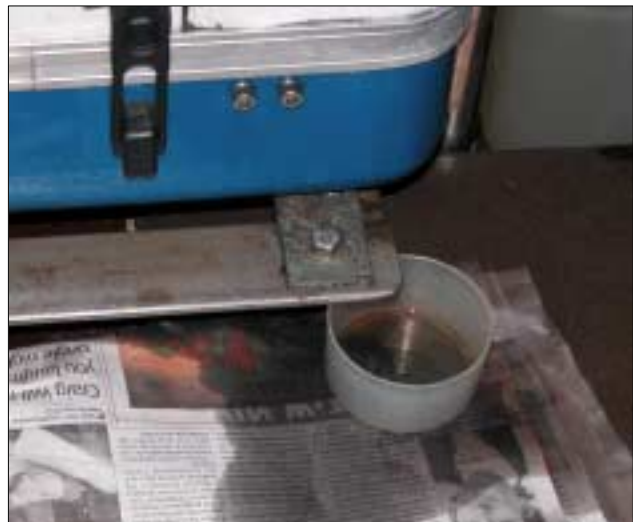
Figure 26. The Panda generator, leaking diesel again. DSCN1091.jpg
