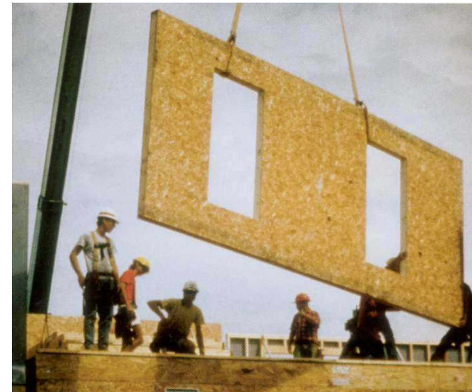
Large panels allow a quick assembly on site . A crane is an essential tool
