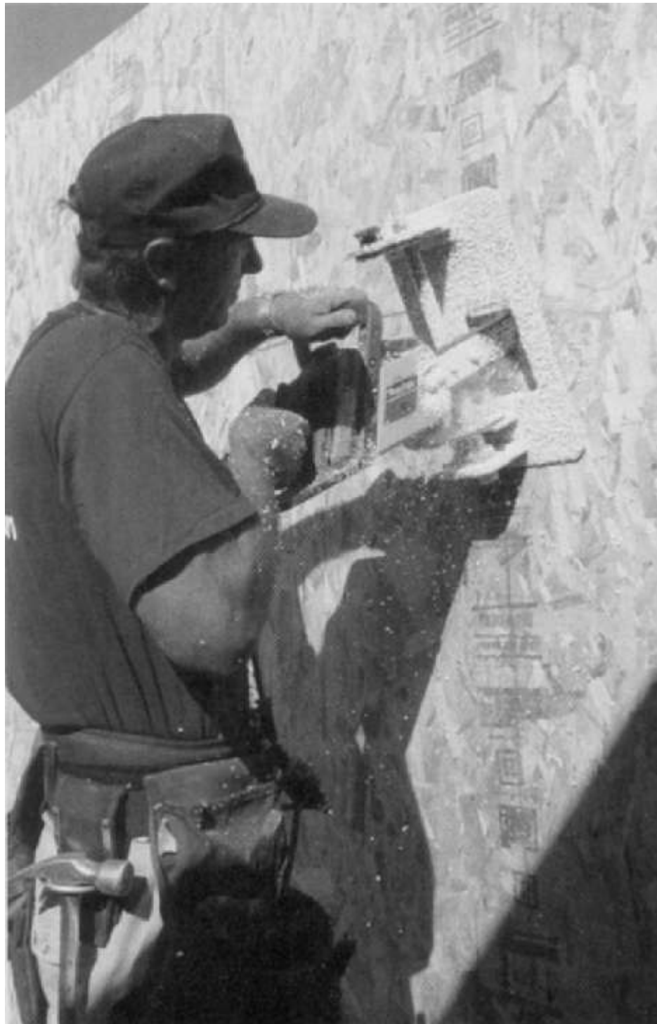
Cutting out a window opening in a SIP panel is a simple, straightforward task.
