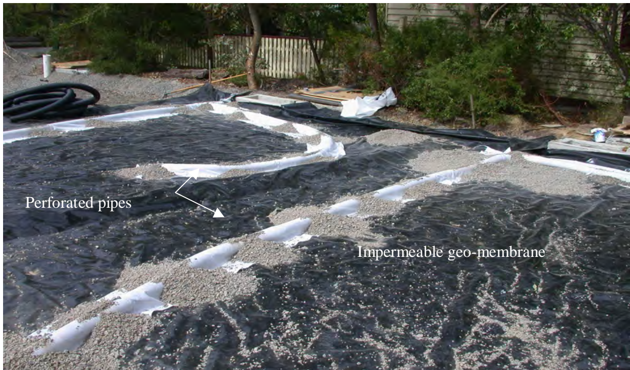
Figure 4.10 The pervious car park during construction at the CERES Environment Park in Brunswick, Melbourne
