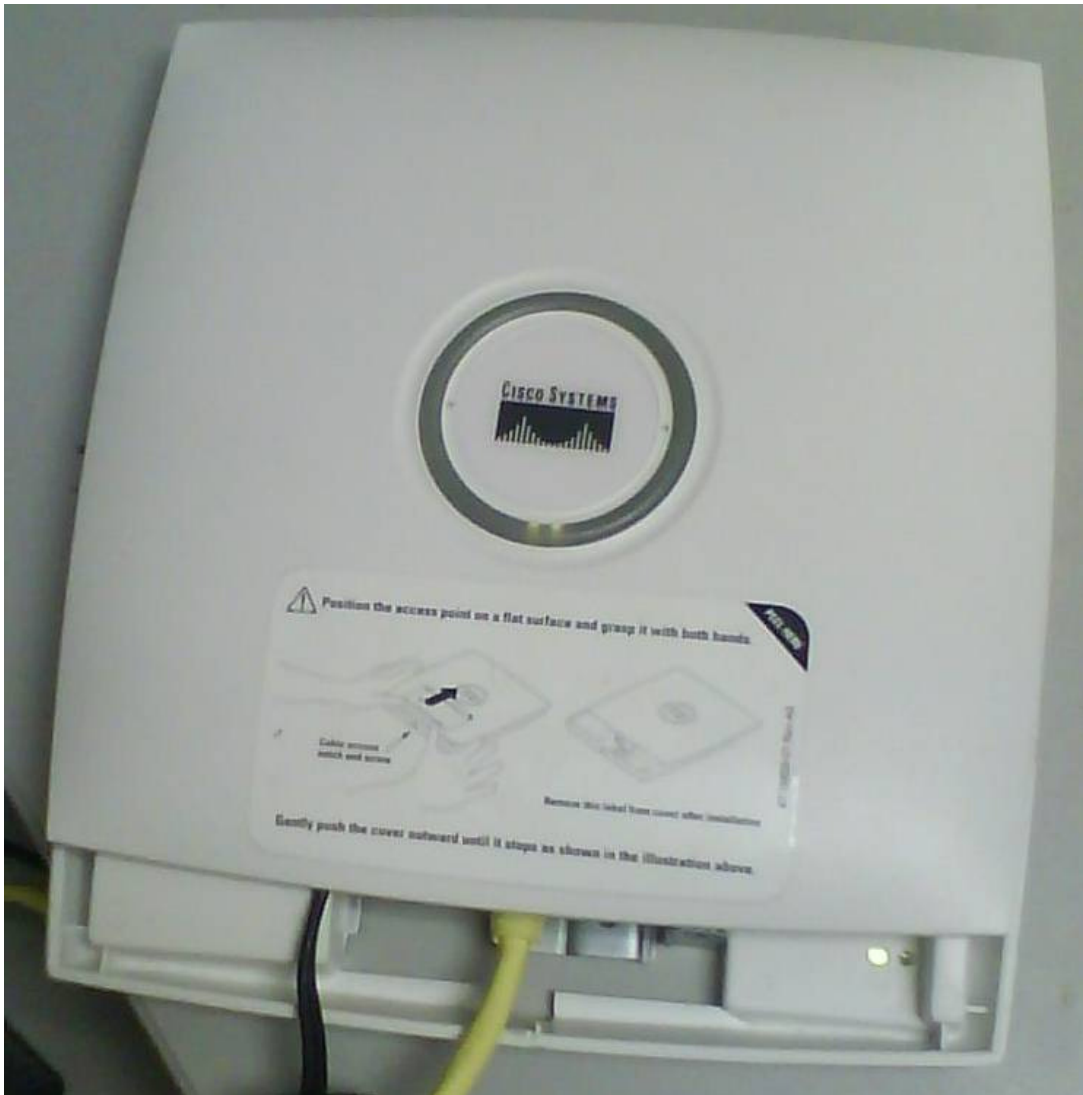
Figure 9-3 Wireless Access Point
