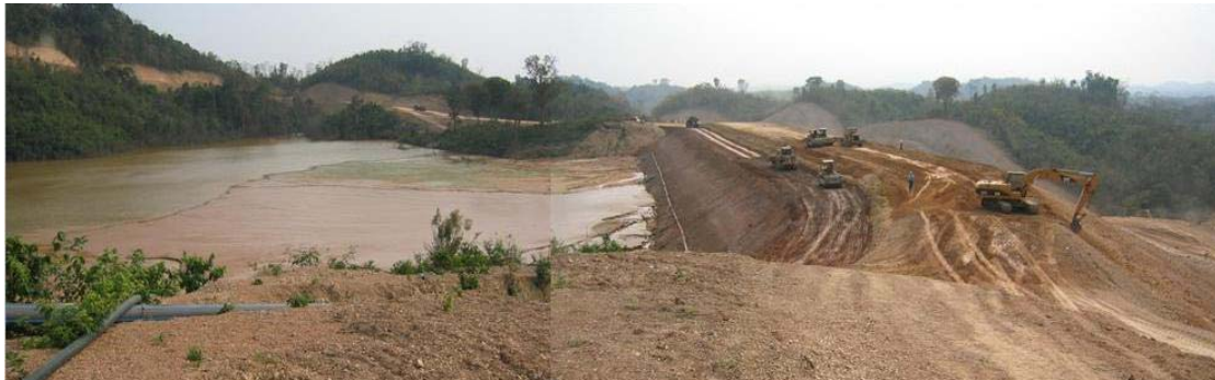
Figure 1. Photograph of a tailings impoundment during a downstream raise of the dam
