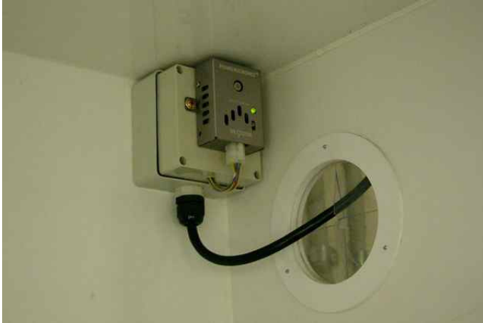
Figure 48: Hydrogen gas detector inside the hydrogen experimental cabinet is connected to the safety system.
