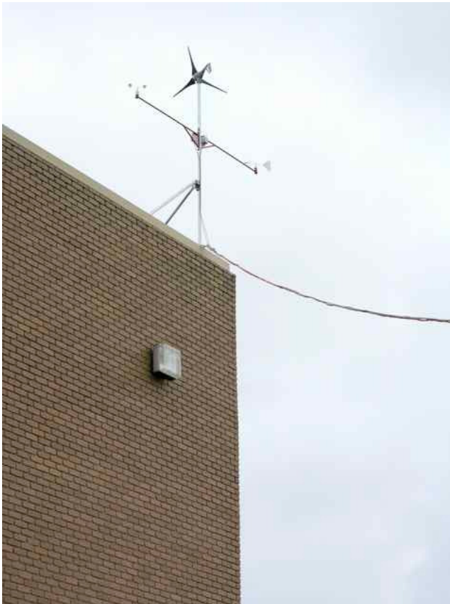
Figure 39: The AIR 403 aerogenerator, anemometer and wind vane installed on Building 253, at RMIT Bundoora East campus. Power line and data cables run into the Renewable Energy Laboratory.
