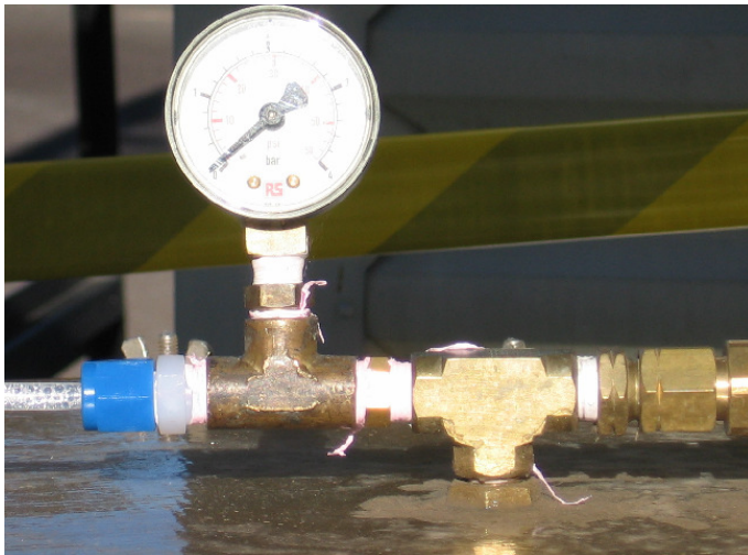
d. Pipe assembly at hydrogen outlet from bottom tank
