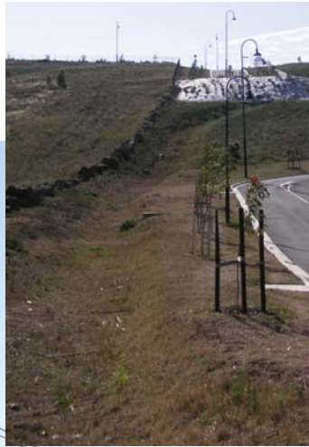
Grass swale does not appear to take run-off from the road.
