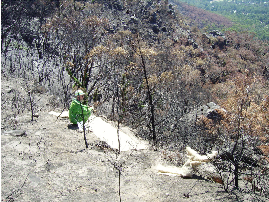
Figure 2-16: Installation of matting post-Mt Lubra fire to minimise erosion on Borya mirabilis field site.
