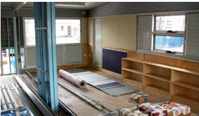
Completed classroom at factory showing cladding left off at module joints and transportation supports (blue steel)
