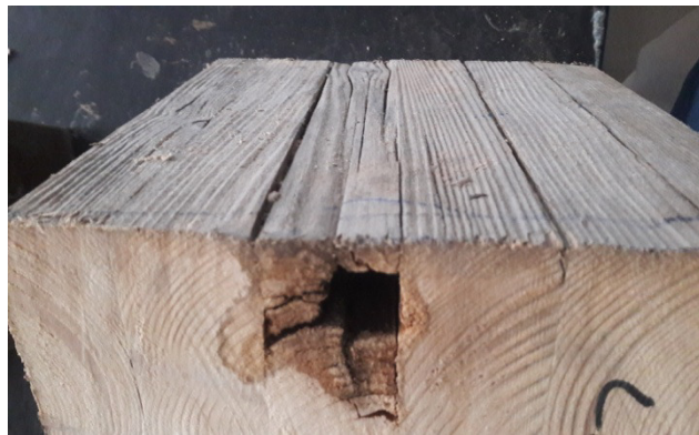
Fig. 6 – Degradation in a cross section
