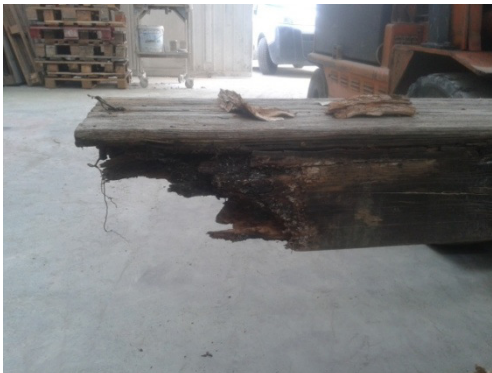
Fig. 7 – Degradation of the beam on bearing
