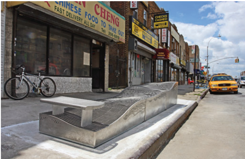
Figure 5.2. MTA commissioned these elevated ventilation units to stay above flooding, Jamaica, Queens. Source: Photo courtesy MTA.
