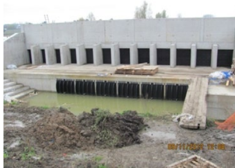
Figure 5 Inlet and outlet sluice configuration in the river side (construction phase) (source: Patrimoniumdatabank W&Z)
