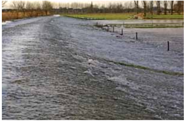
Figure 1.4. Scheldt water flooding over the overflow dyke in the Paardeweide FCA
