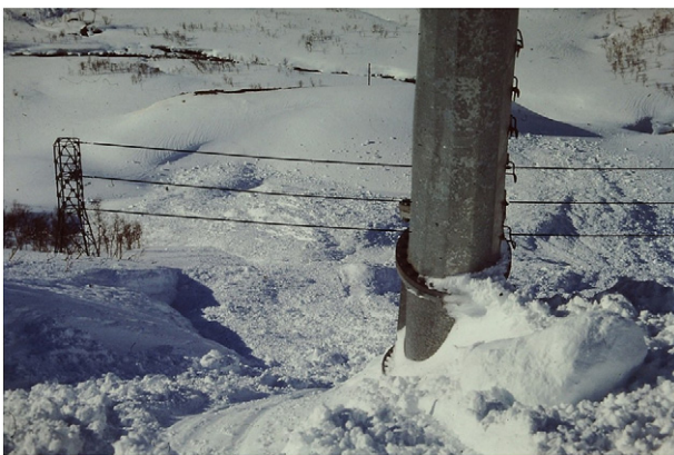
Fig. 22. View from the Y-mast (now LC54) down to the catching dam and the transmission line assembly after the avalanche event 1989-03-04. The cables were 4 m apart and their diameters were \phi 34 mm. The concrete wedge (LC321) is the snow covered hump just left of the mast.
