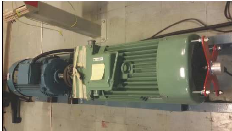
Figure 7.1: Motor Generator set.
