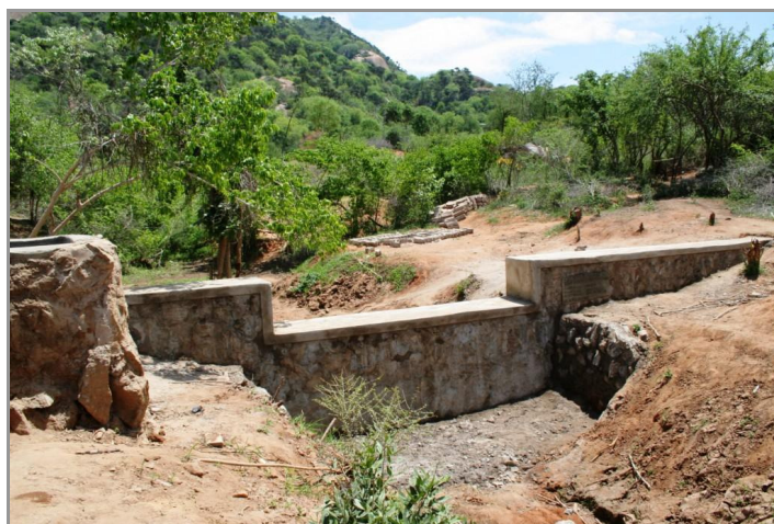
Figure 1.3 A new build dam without any sand accumulated behind it yet. The spillway is in the middle of the dam.
