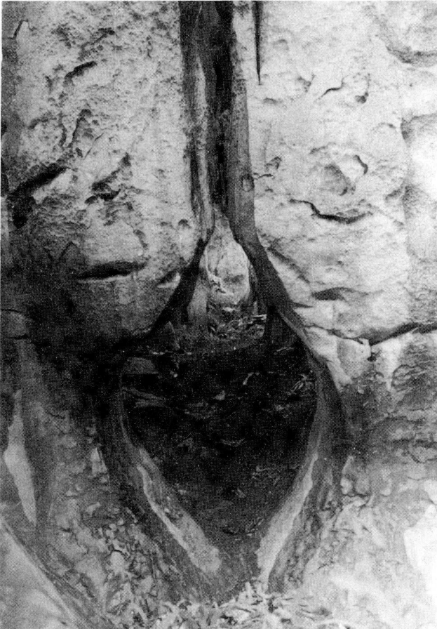
Fig. 5 - Horizontal subsoil erosion tube.
