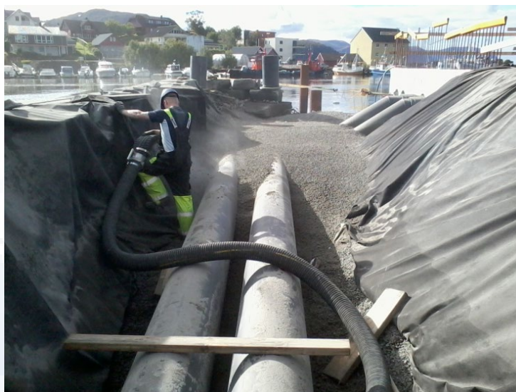
Figure 7-11 Pipelines for supplying water used as a heat source for heat pumps in a district heating system in Ulstein © Øyvind Amdam, Ulstein municipality
