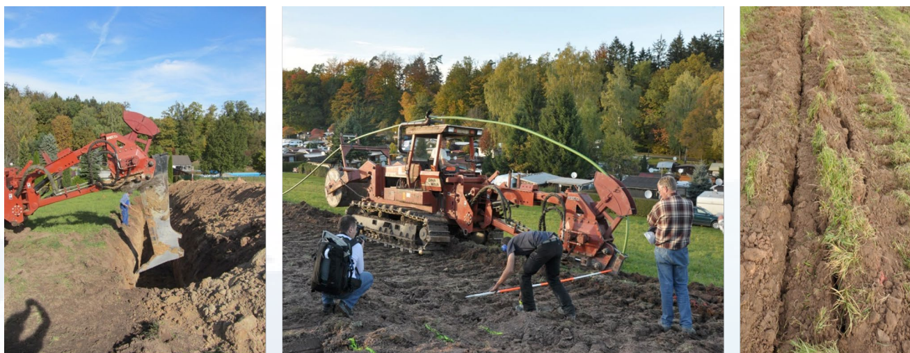
Figure 7-4 Thermal activation of the agricultural field in Wüstenrot © HFT Stuttgart
