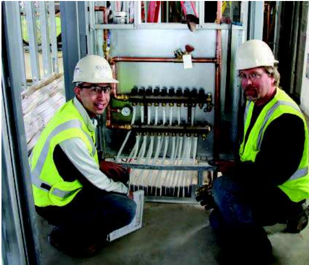
Fig 3: Manifold in Flush-mounted Wall Cabinet
