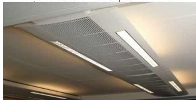
Fig 2: Radiant cooling panel attached to ceiling
