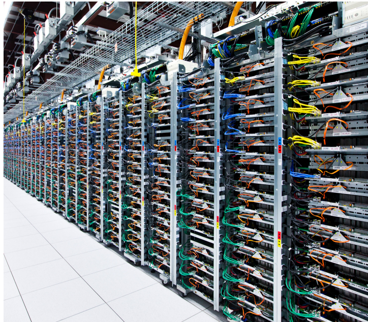
Figure 2.1: Data centres need significant amounts of wiring (image from Google)
