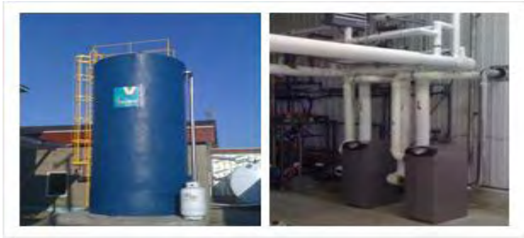
Figure 2-10 Treatment unit of anaerobic digestion of the Dairy industry La Vachea Maillotte Cheese Dairy [156].
