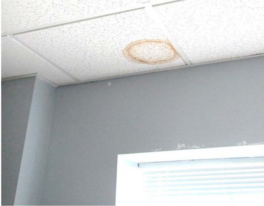
Water-damaged ceiling tile
