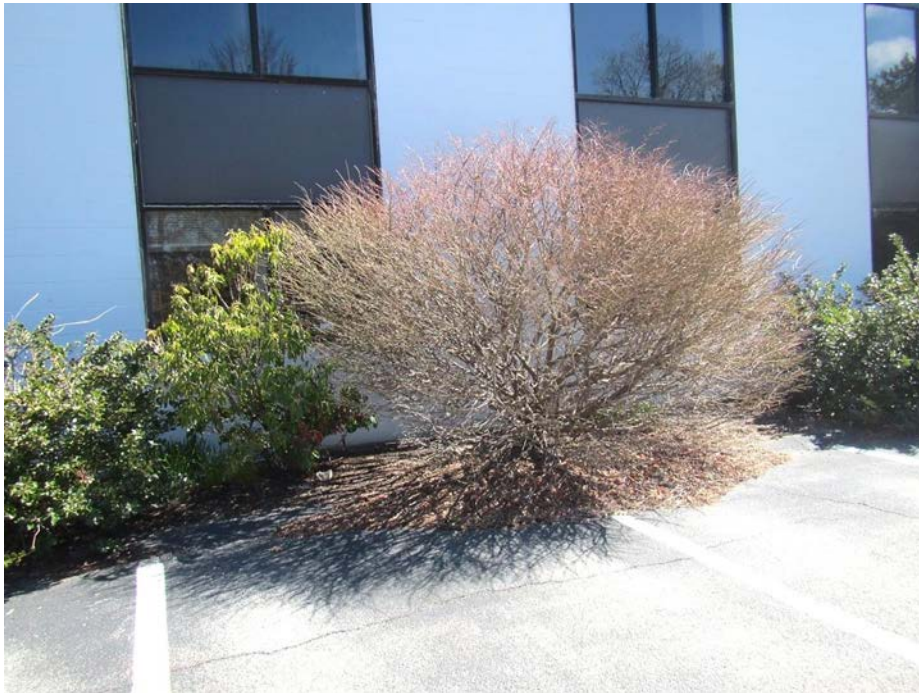
Plants in contact with foundation
