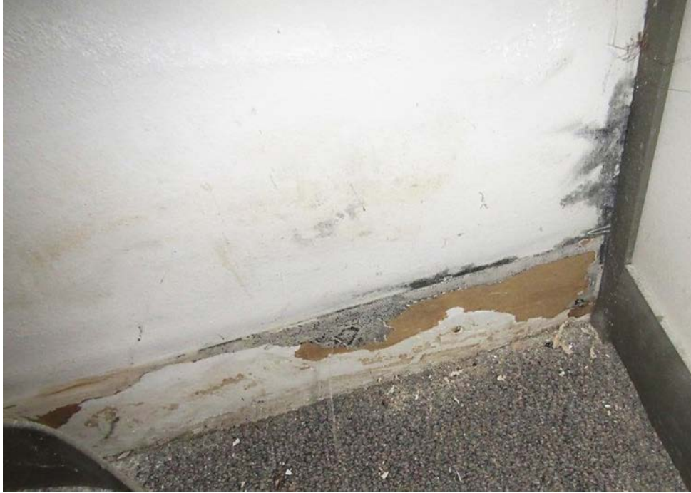
Water-damaged/mold stained wall and removable coving indicating past moisture
