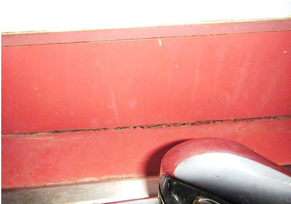
Open and stained backsplash at kitchen sink
