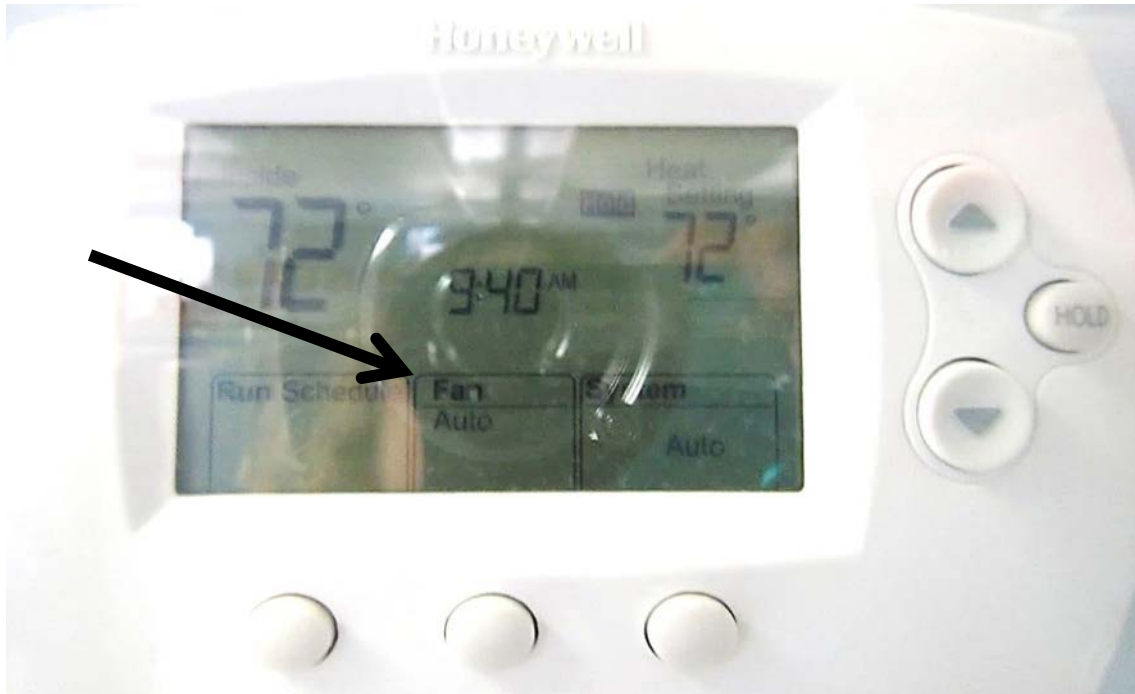
Thermostat showing fan in “auto” mode (arrow) and incorrect time
