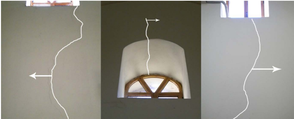
Figure 7. Structural cracks in the interior of the mosque
