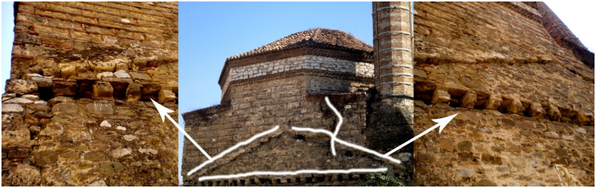
Figure 6. Structural cracks in the north façade
