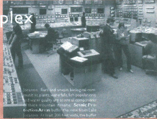
Reactor Control Room
