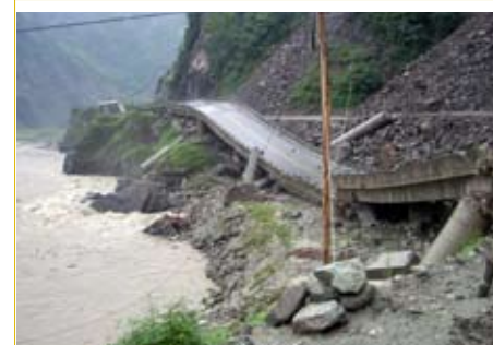
Wenchuan earthquake - Collapsed motorway bridge along the Min river in Ying Xiu Town middle school in Ying Xiu Town.
