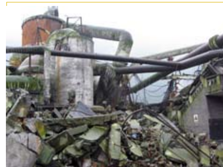
Natech accident: Damage in a fertilizer plant as a result of the Wenchuan earthquake in China.
