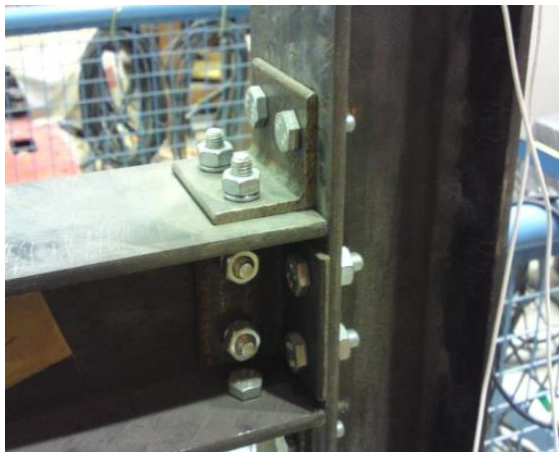
(c) Beam-column joint.
