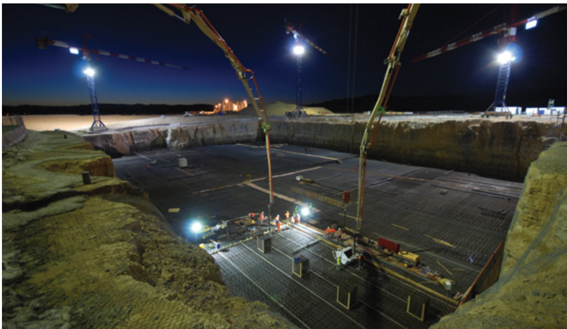
Pouring concrete in the Tokamak complex at 5:00am, August 2011 (courtesy of the ITER IO)
