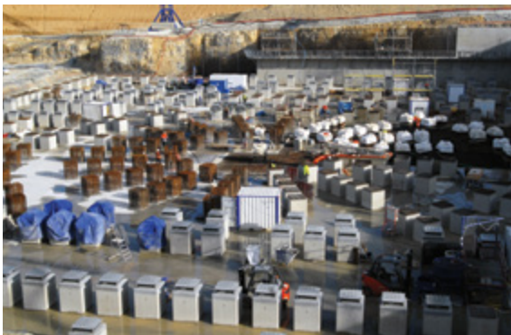
A panoramic view of the Tokamak complex in late December 2011 showing the progress of the anti-seismic bearings
