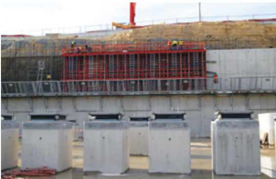
View of the four plinths with anti-seismic bearings on top
