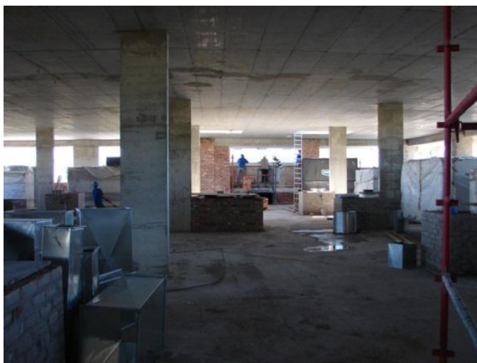
Access route through unsafe construction area of some staff for security installations in basement.
