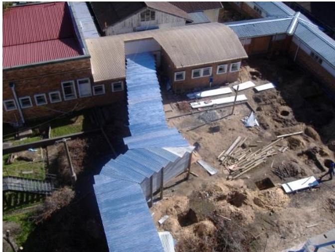
Aerial view of temporary walkway which had to be used by staff and to connect wards with services (food, linen and stores)
