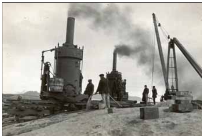
7.11 Channelers at work at No. 3 Quarry in 1912. Note the running water. (Source: pol02988, Polar Museum, Tromsø.)
