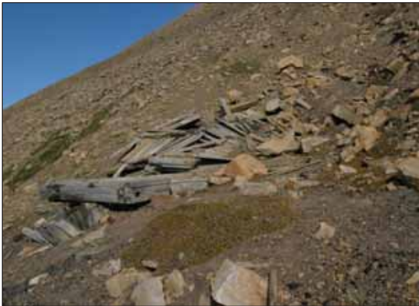
3.5 Timbered opening (1b) collapsed under creep. (Photo: L. Mishkar, LASHIPA 1, 2004).
