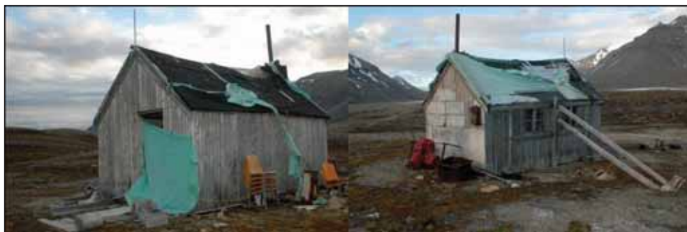
4.82 The Scottish hut in Gips Valley had seen frequent re-use. (Photos: D. Avango, LASHIPA 3, 2006.)
