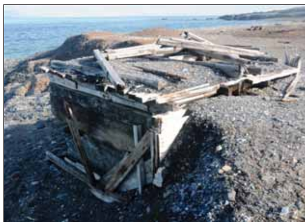
4.37 Concrete shaft (3) with collapsed shafthead frame at the Icefiord Zinc and Lead Mine. (Photo: P. Leminen, LASHIPA 9, 2010.)
