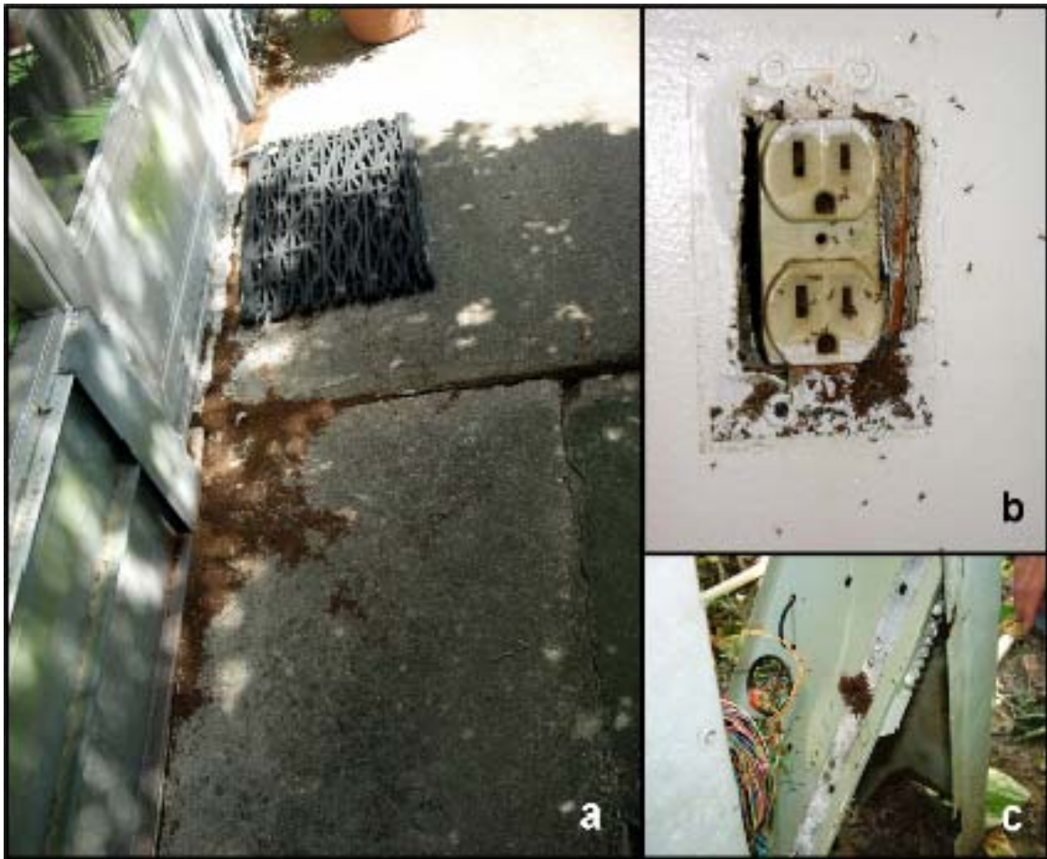
Figure 8.1. These pictures represent the large numbers surrounding structures and the potential electrical damage of P. sp. nr. pubens . A) Taken in June, this picture demonstrates the remarkable numbers of a graveyard of P. sp. nr. pubens workers prior to a treatment. B) P. sp. nr. pubens workers have shorted out this outlet. C) P. sp. nr. pubens have shorted out this electrical unit located in a the backyard in the Deer Park, TX neighborhood. These shortages had created several power outages for whole streets in the neighborhood.
