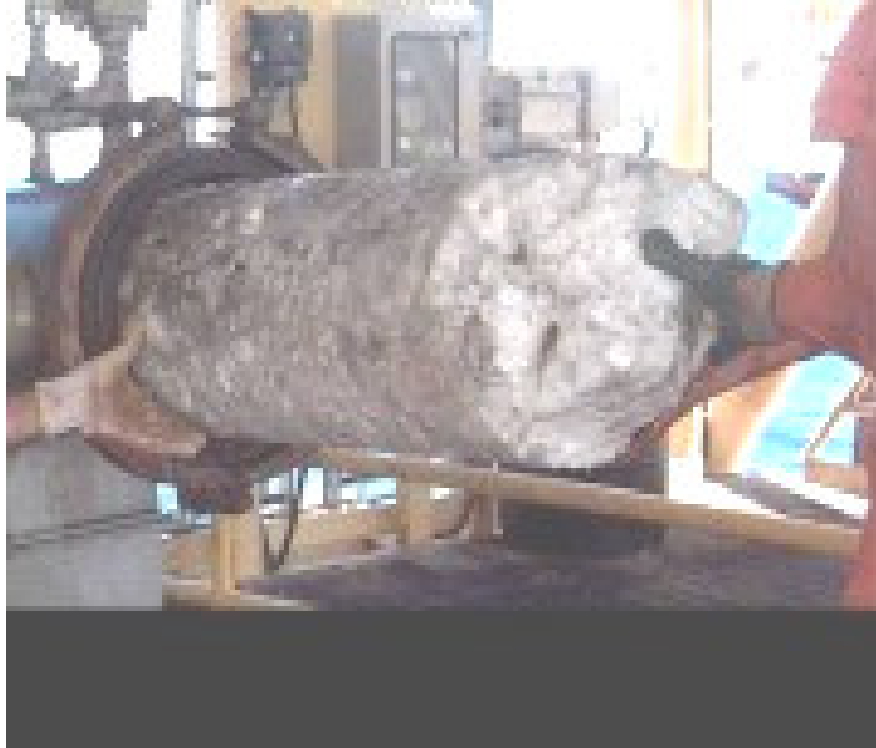
Fig. 2.3—Formation of gas hydrate plugs a subsea hydrocarbon pipeline. 25
