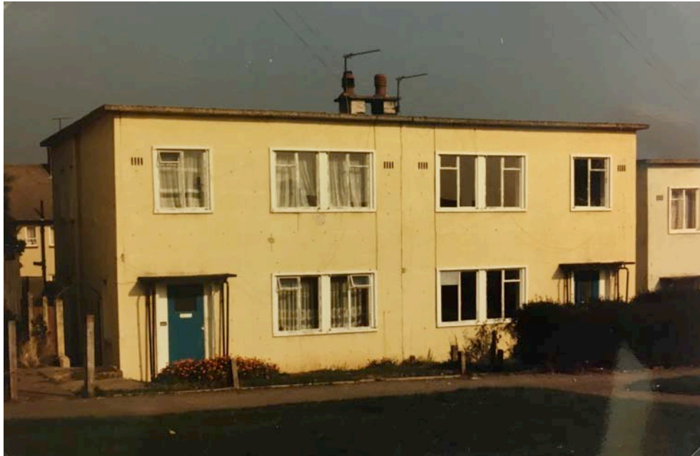
Figure 8.18 The flat-roofed Orlit House c. 1990. (Photo by Paul Francis, Airfield Research Group)
