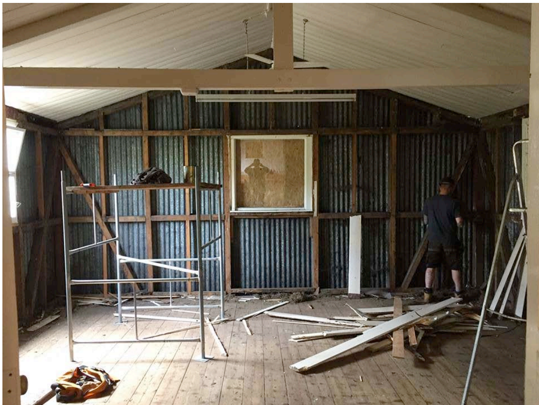
Figure C.2 Dismantling of the Girton Women's Institute Hut shows the original corrugated metal sheets set to the timber frame. (Taff Gillingham and Great War Huts)
