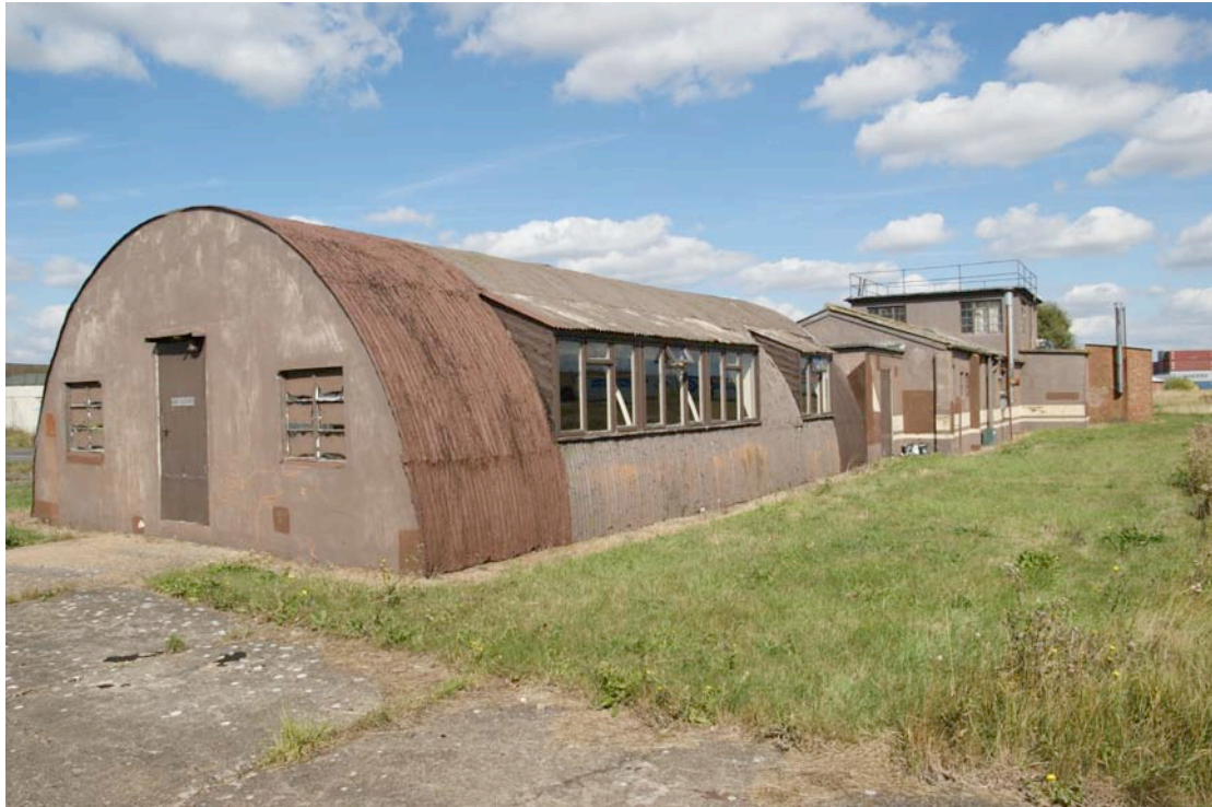
Figure 7.7 A Nissen hut with dormer windows located at RAF Alconbury. Photo by Paul Francis (Airfield Research Group)
