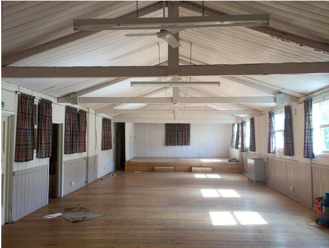
Figure C.1 Interior view of the Armstrong Type Plan Hut prior to dismantling for its move to the Great War Huts site. Originally built in October 1914, it was repurposed as the Girton Women's Institute Hut c. 1920. (Taff Gillingham and Great War Huts)
