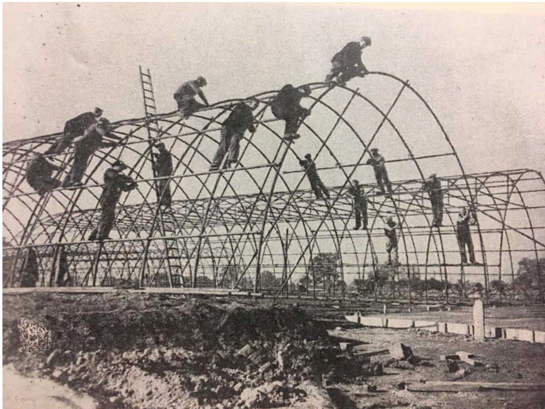
Figure 7.10 Workers erect two Iris Huts for storage and workshop requirements at a military camp in 1942. The Architects' Journal , (19 November 1942)
