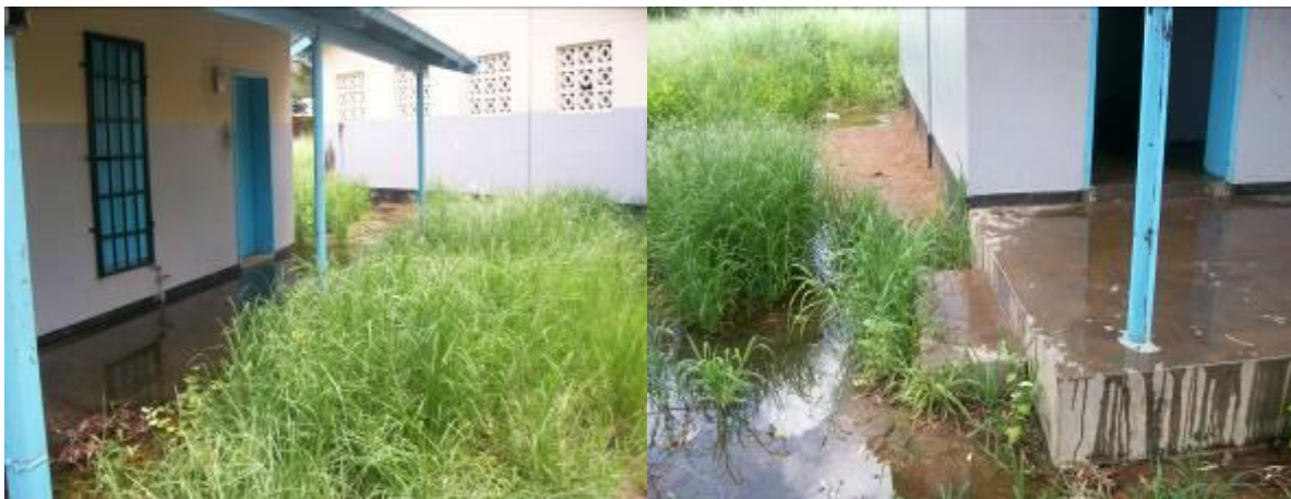
Plate B6.2 Overgrown grass behind classrooms and around toilets and leakages
