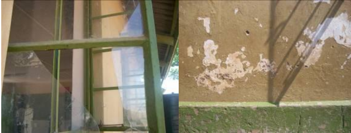
Plate A6.2 Broken window and peeling paint on classroom walls
