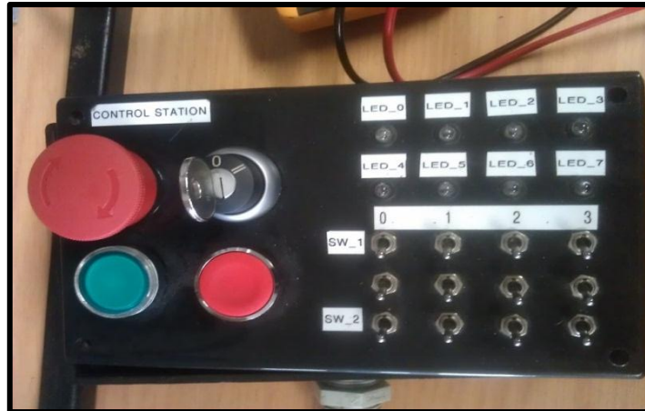
Figure 4.18: Control Box for BOW system
