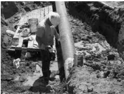
Fig 5: Damaged underground pipeline
