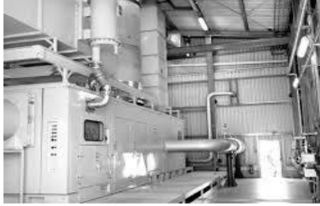
Enclosed Gas Compressor Building
