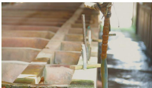
Figure 45: Water dripping from a valve. (Inhalation, 2010)
