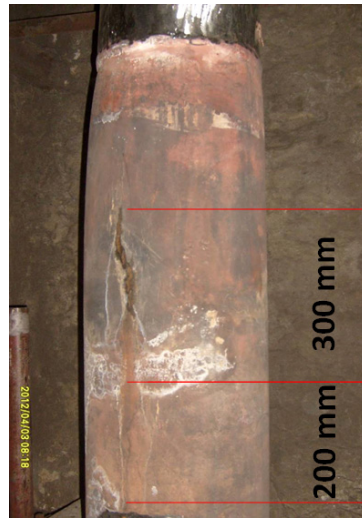
Figure 5: Determination of damage by visual inspection.
