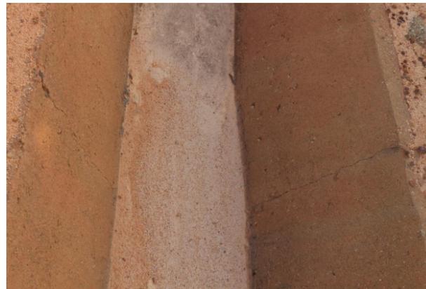
Figure 20: Crack on drainage networks facility, made up from thin plain concrete cross section.
