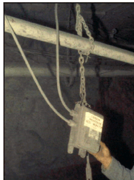
Figure 13.—CO fire sensor mounted in mine entry.
