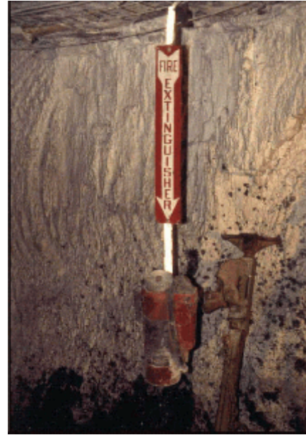
Figure 8.—Dry-chemical portable fire extinguisher mounted on the rib.
