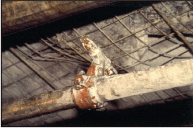
Figure 14.—Sprinkler system installed in mine entry.
