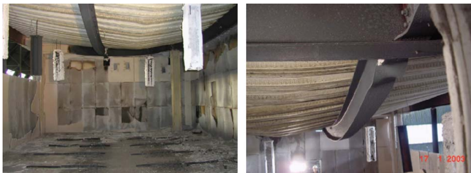
Fig. 9. Compartment after fire, residual deformation 925 mm, no local collapse of structure.
