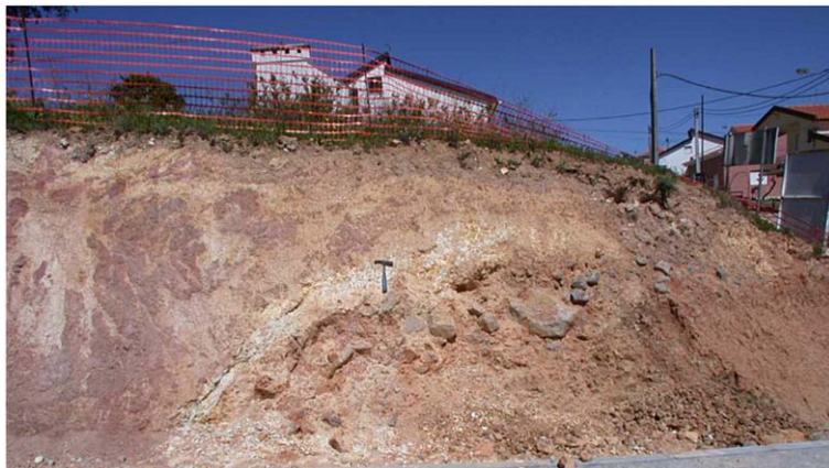
Fig. 7. Outcrop oriented E–W, at Vila Velha de Ródão, showing the metamorphic basement thrusting the Cenozoic. The hammer indicates the fault plane.
