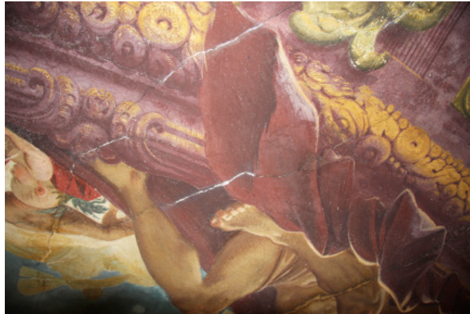
Image 96: Cracks of the false ceiling
