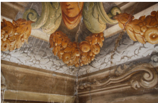
Image 77: Crack of the false ceiling in the ballroom
