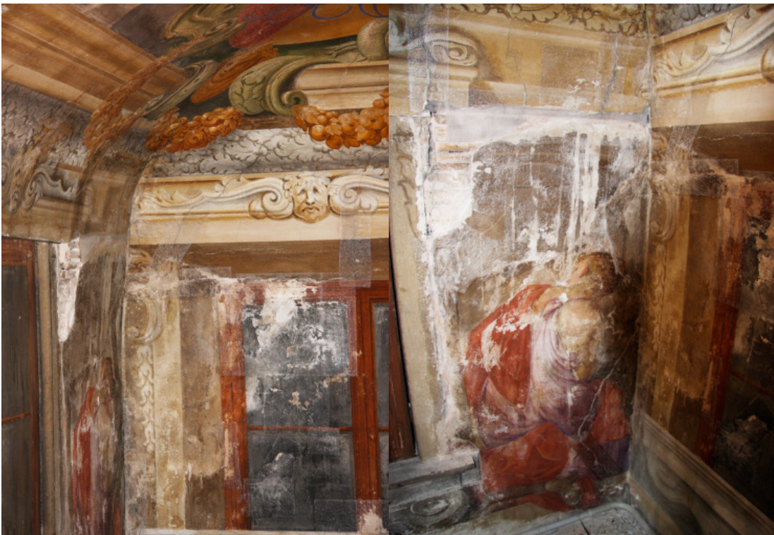
Image 100: Decay for seepages
