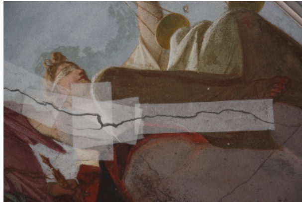
Image 76: Crack of false ceiling in the portego
