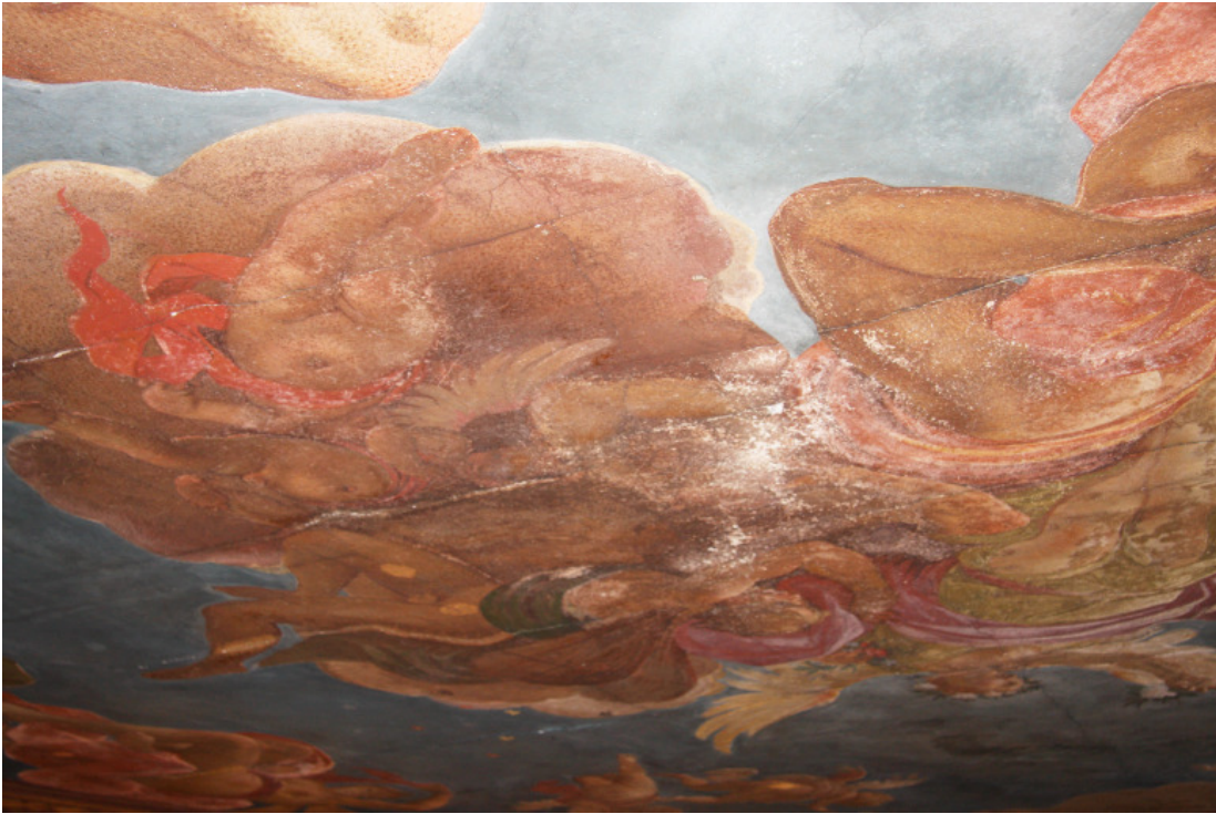
Image 99: Superficial erosion, cracks and lacuna
