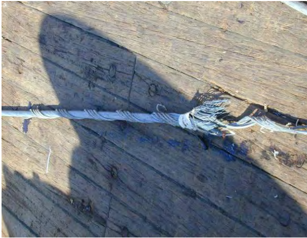
FIG. 4.21: The broken cable termination.
